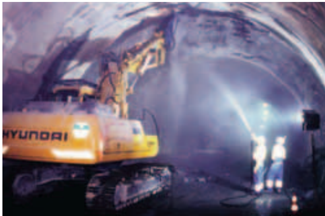
Photo 3 Lavage à haute pression High-pressure washing
