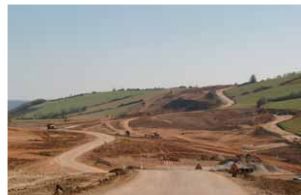
Emplacement de la future gare de péage Location of the future toll station
